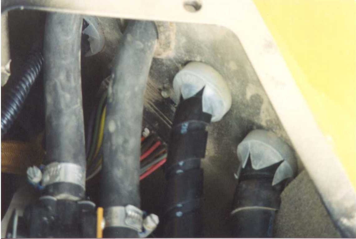
Hoses into evaporator box with clutch wire in background.
